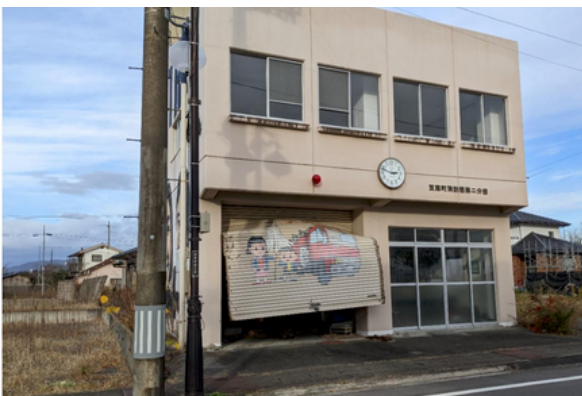
A firehouse in Futaba town with a broken clock
